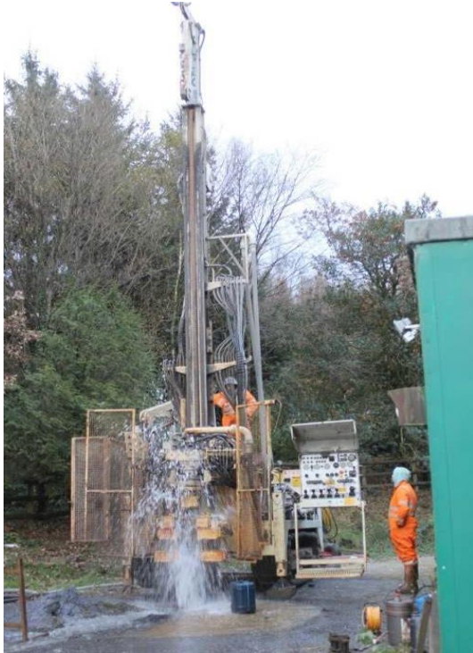
Figure 1. Drilling into old mine workings at Crynant, South Wales. (Photo courtesy of WDS Green Energy Ltd)
