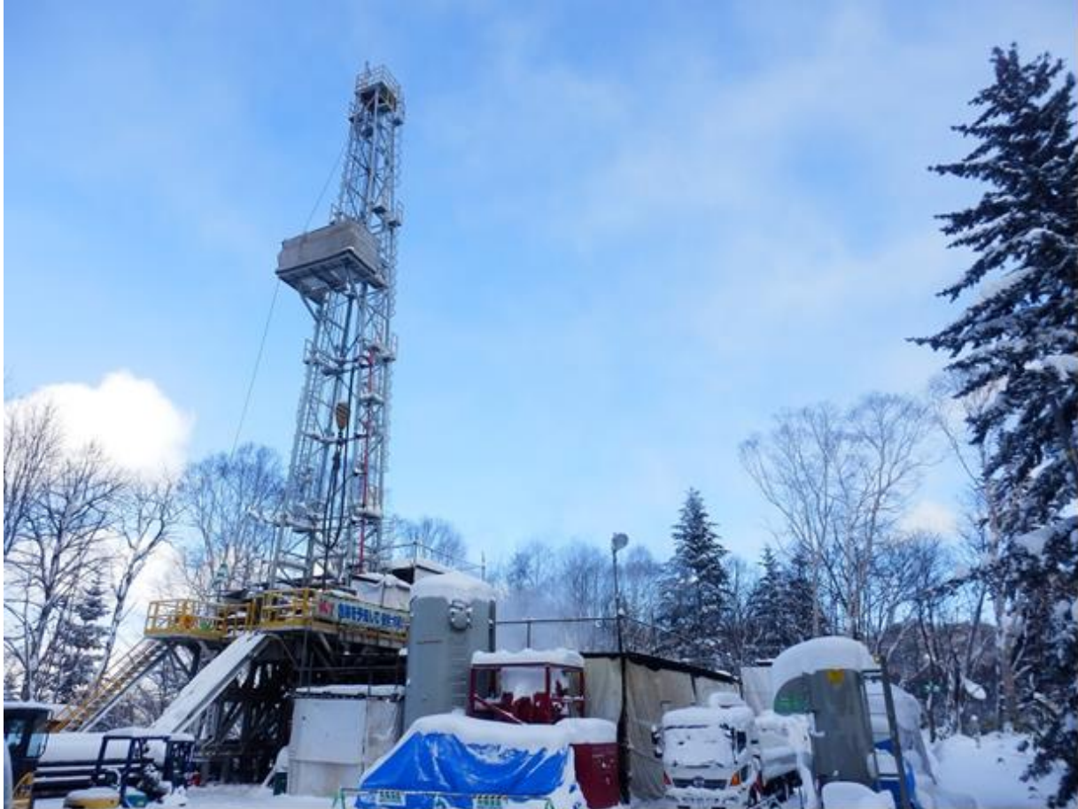
Figure 14.1 Drilling of an investigation well at the Toyoha field in Hokkaido, Japan, conducted by JX Nippon Mining & Metals Corporation (Photo courtesy of JOGMEC on 21 November 2012)
