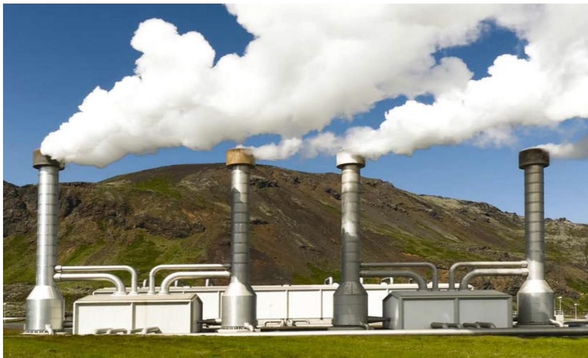
Figure 12.1 Nesjavellir geothermal power plant.
